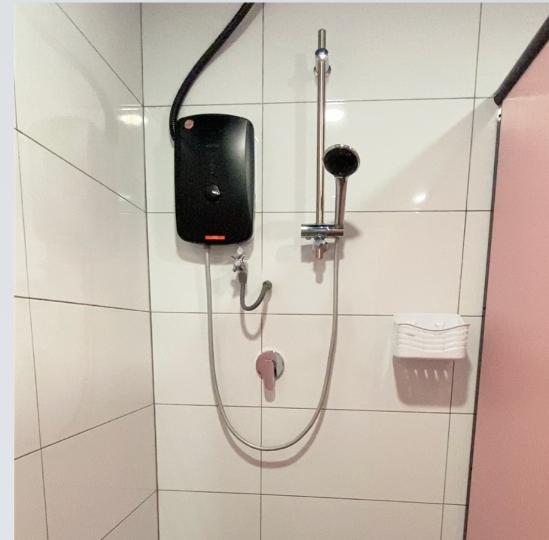
Hot Shower Facility
