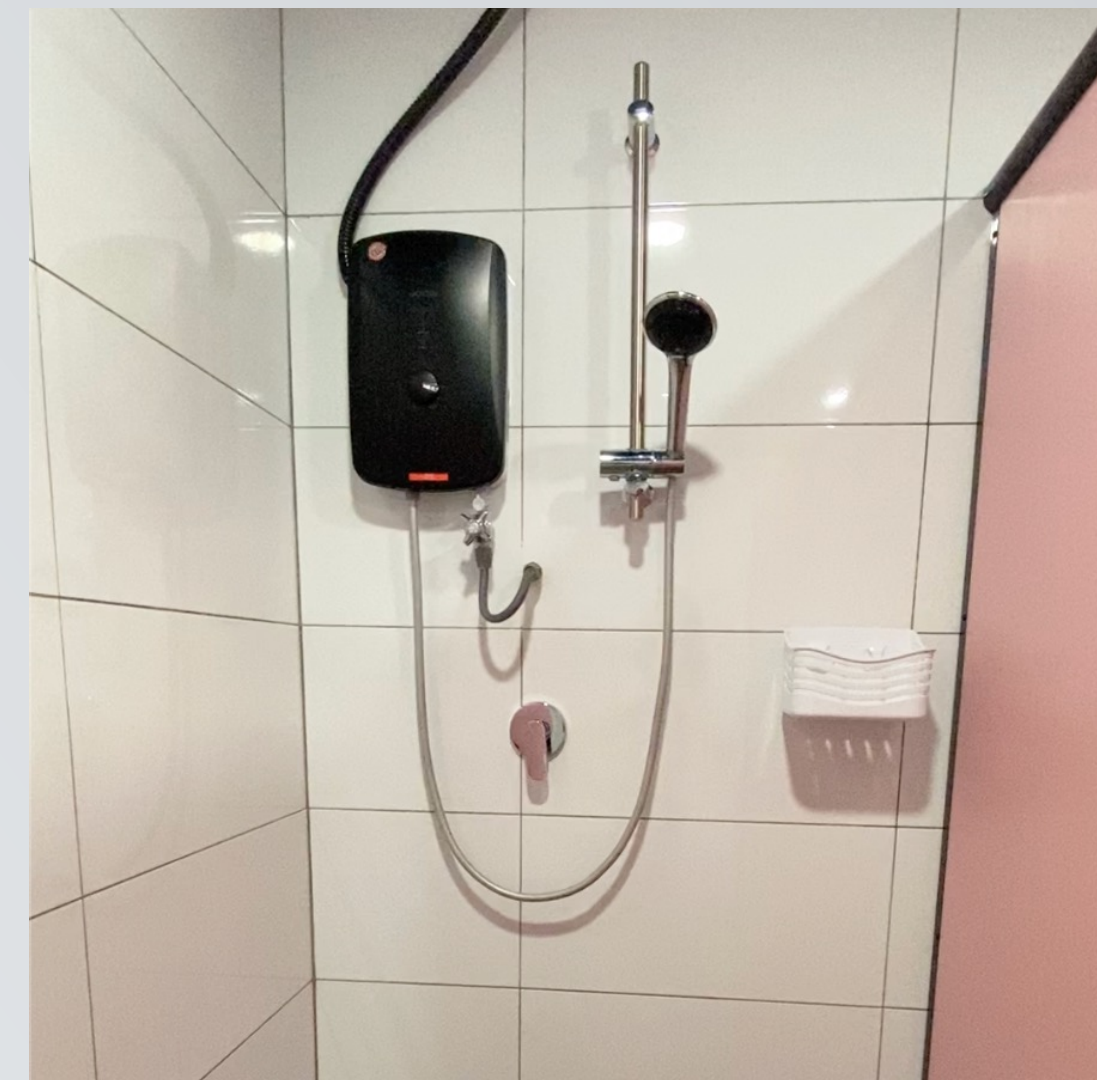
Hot Shower Facility
